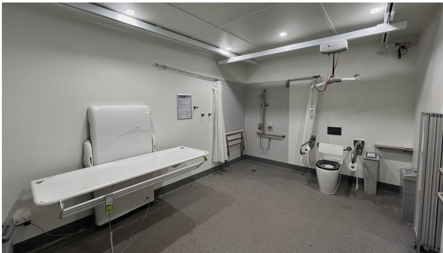
Above: Interior of the Changing Places facility.
