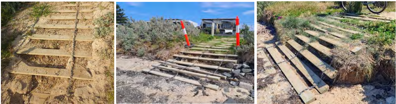
Figure 6-1 Erosion undermining of sand ladders – safety issue
